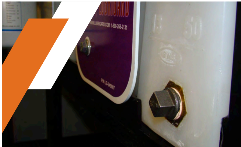
SEE FIG.5.A.1 – STEEL FRAME PLATE BAR WEDGED BETWEEN THE POLY TANK AND THE STEEL PUMP
